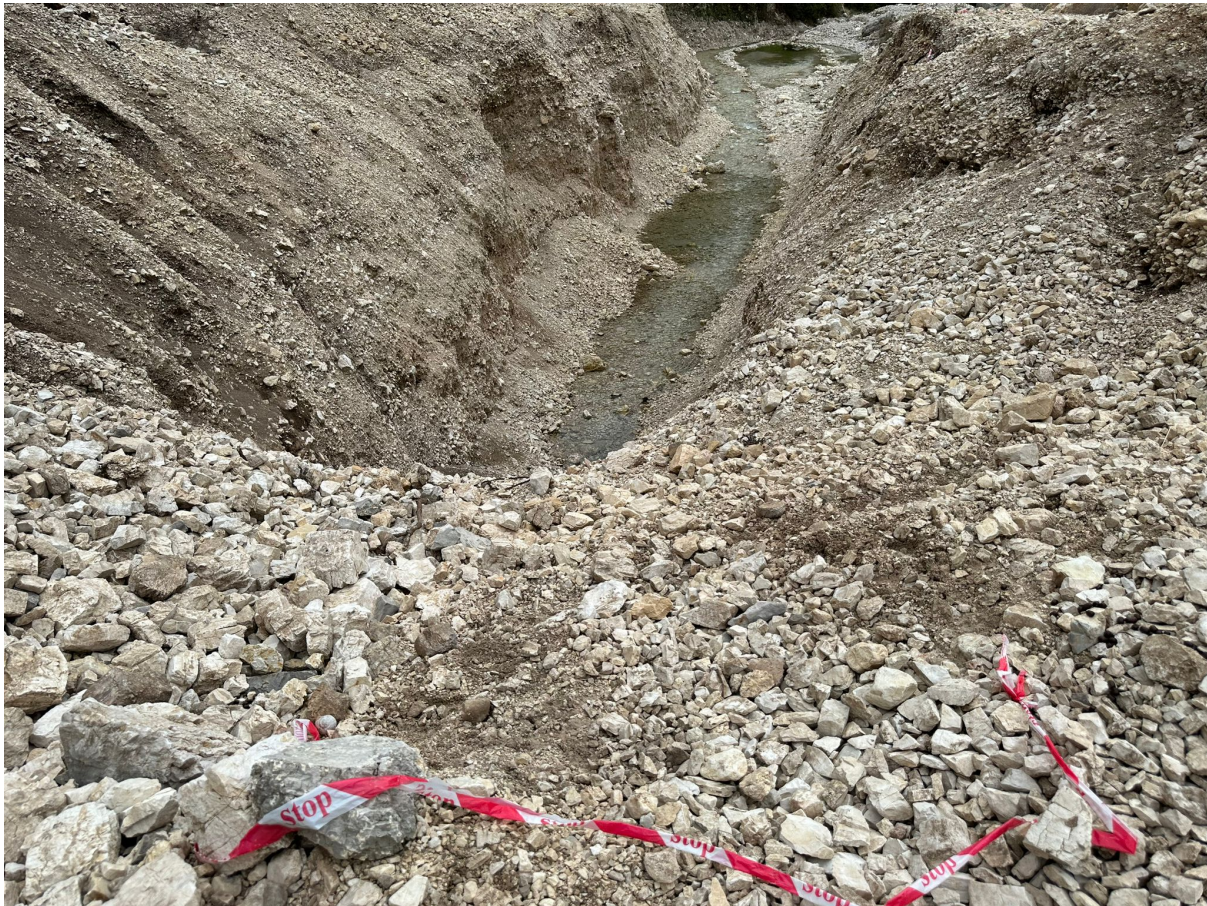
Figure 7: The 5-6 meters deep channel of the intake on the left side of the Shushica River © U. Eichelmann
