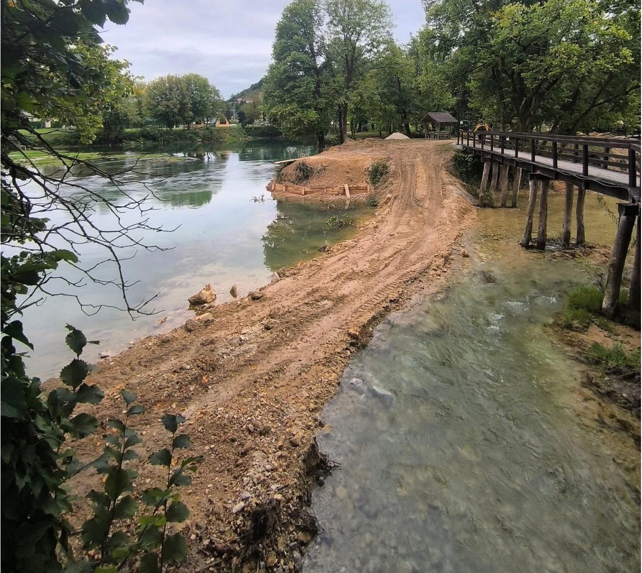
Construction of a new river crossing within the Una Valley. (picture: Anes Halkic)
